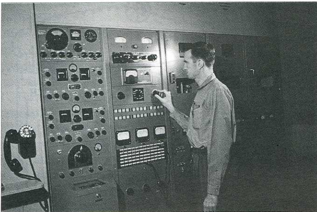
An engineer at the monitoring and control panel
